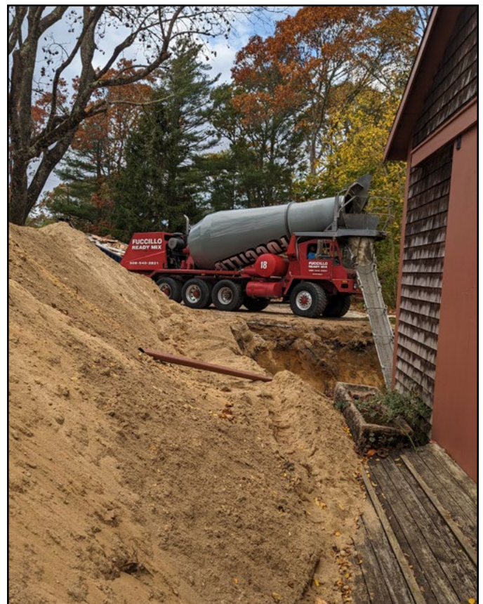
A cement truck, operated by Fuccillo Ready Mix, pours concrete into a newly dug foundation at the former site of HSSC's Fire Museum. The basement of the new building will be a climate controlled collection storage space. Courtesy of the Historical Society of Santuit & Cotuit.
